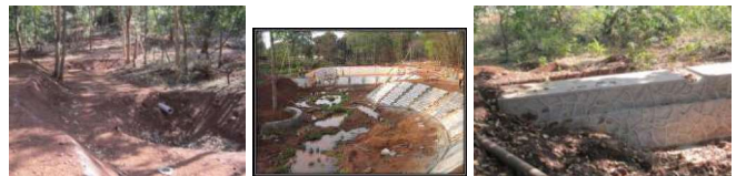
RWH structure for ground water augmentation in the area
