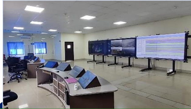
Integrated Command Center to monitor
