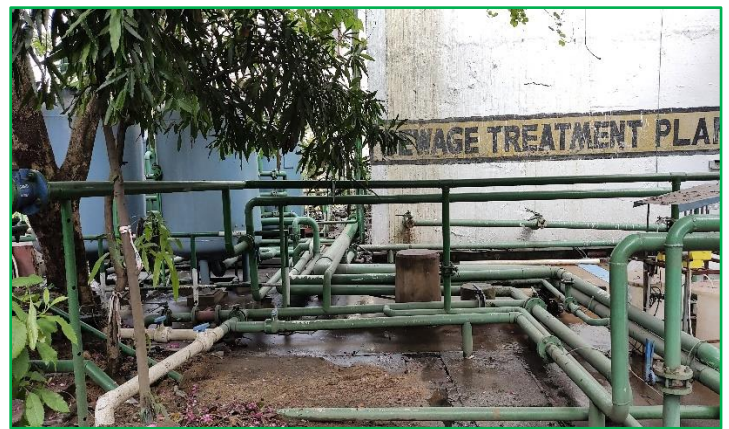
Sewage Treatment Plant (1000 KLD)
