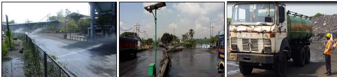
Use of Fixed & mobile water sprinklers in area
