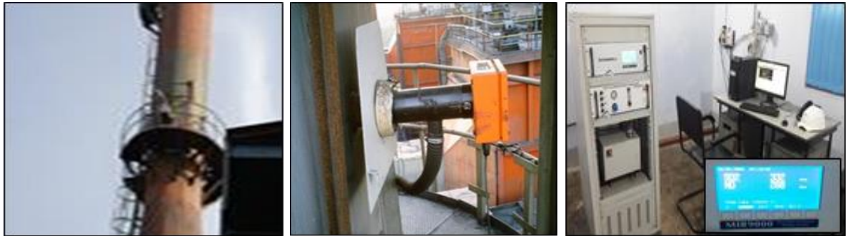
Continuous Emission Monitoring for Power House for PM, Sox & NOx data
