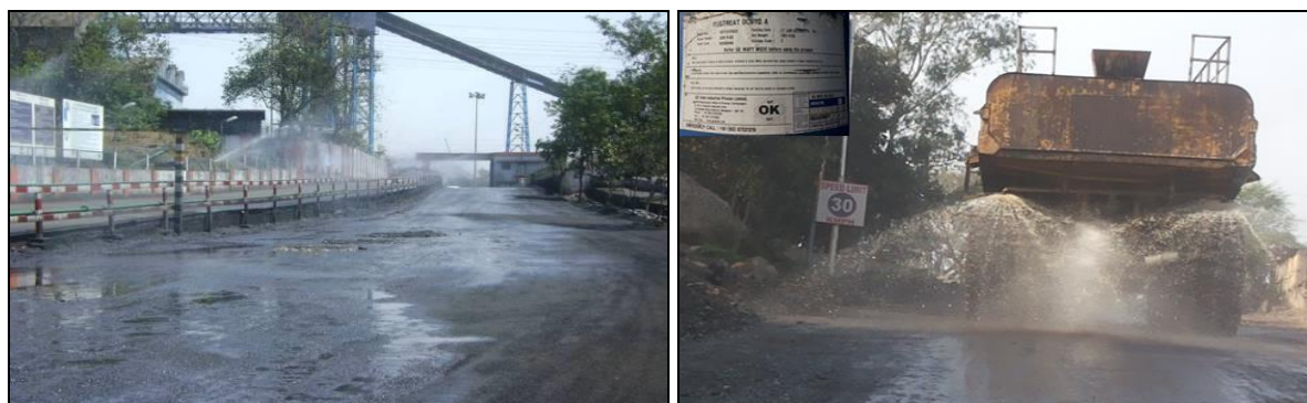
Fixed and mobile water suppression system
