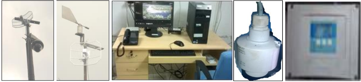
Online Effluent Monitoring System installed at site (Power Plant)
