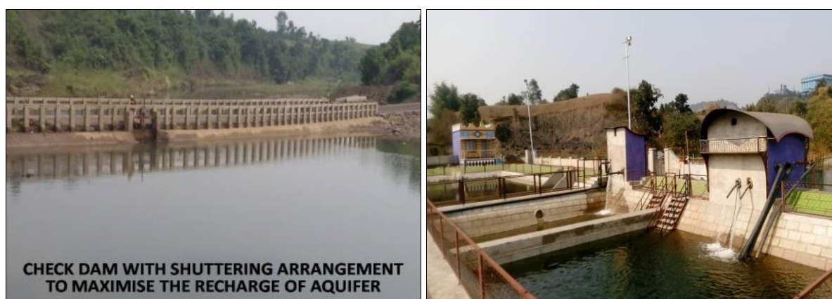
RWH cum drinking water project at Duni village
