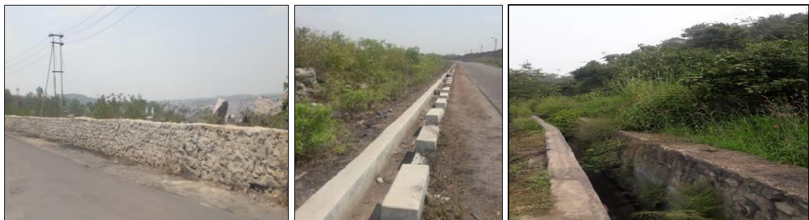
Toe wall & garland drain in the area
