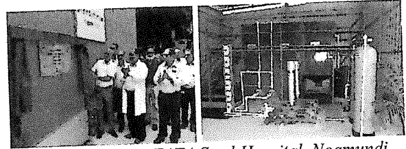
10 KLD ETP at TATA Steel Hospital, Noamundi
