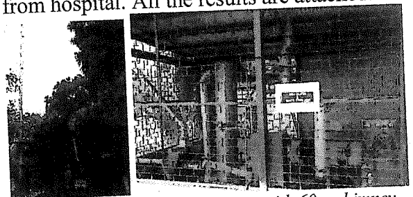
Double chambered incinerator with 60m chimney
