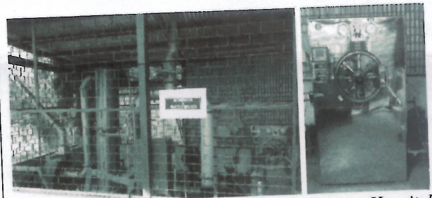
Double chambered incinerator & autoclave at Hospital
