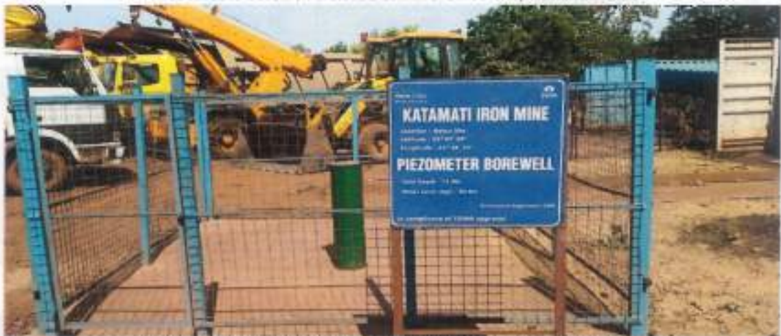
Piezometric borewell installed at METSO Office site, Katamati Mine
